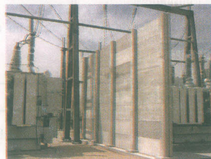
Fig. 2: firewall in electric substation
