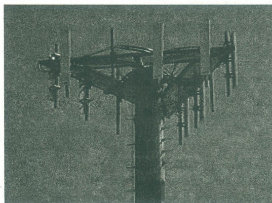
Fig. 7: Top of a cellular radio tower
