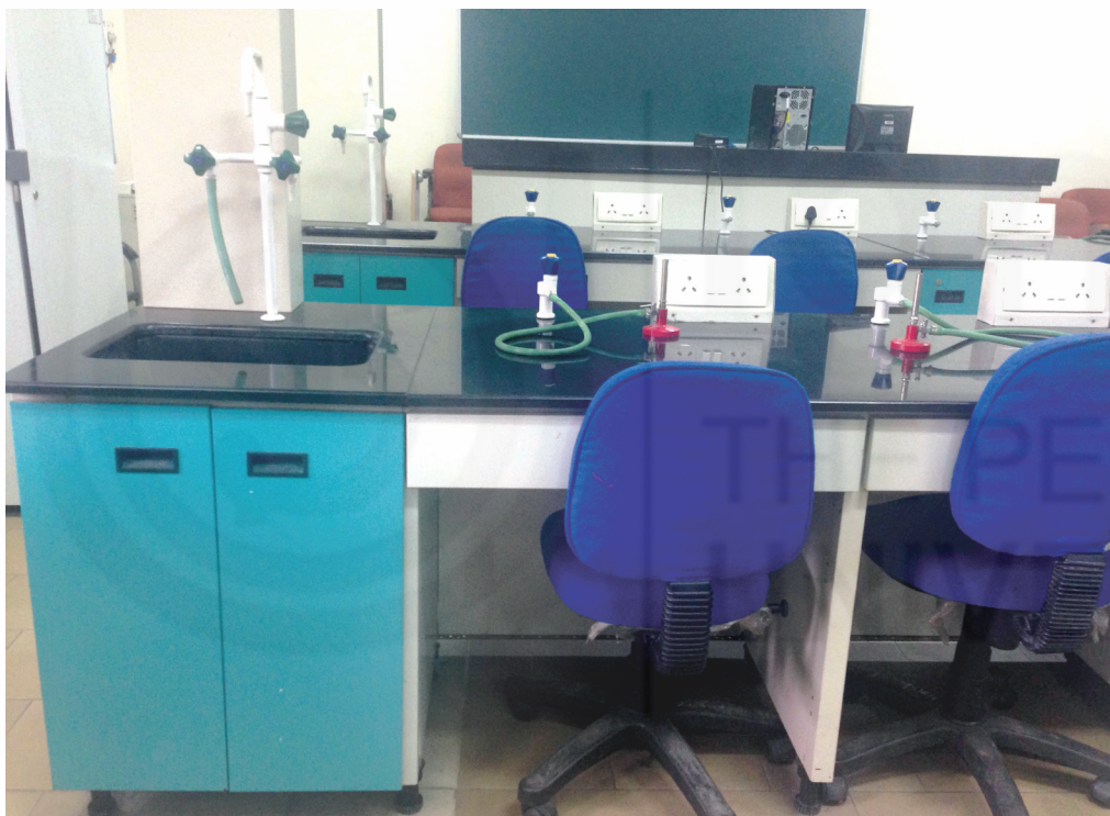
Fig. 2.7: Proper placement of electricity, gas and water outlets on the work bench.
